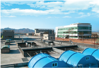
GIC wastewater treatment facility
